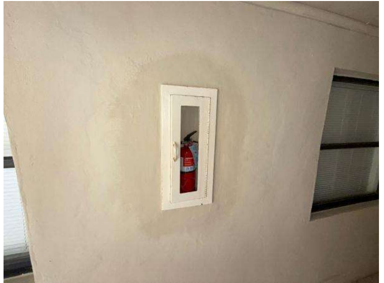
Photos / Fire Protections
