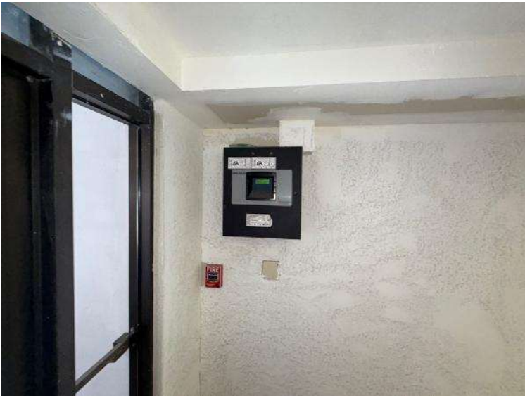
Photos / Fire Protections
