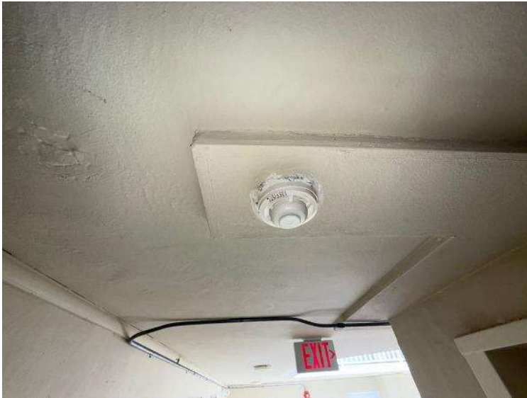
Photos / Fire Protections
