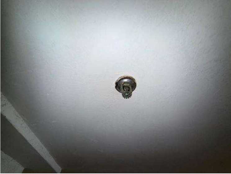
Photos / Fire Protections
