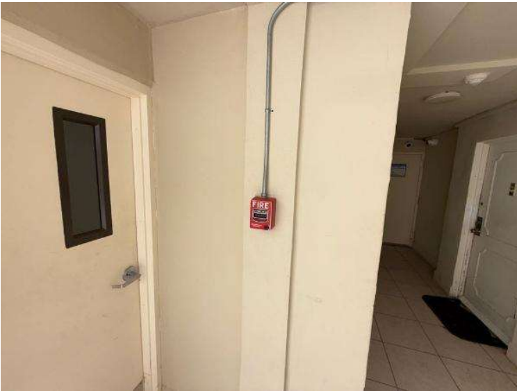
Photos / Fire Protections
